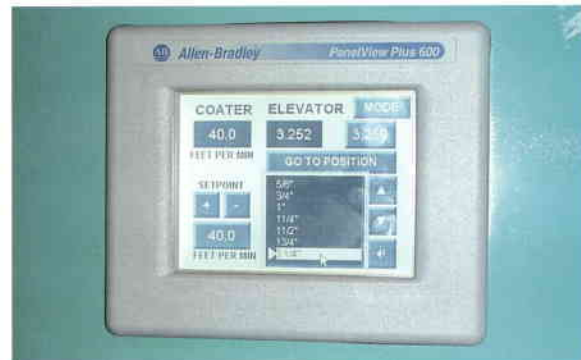
Automatic Elevator Control Panel
